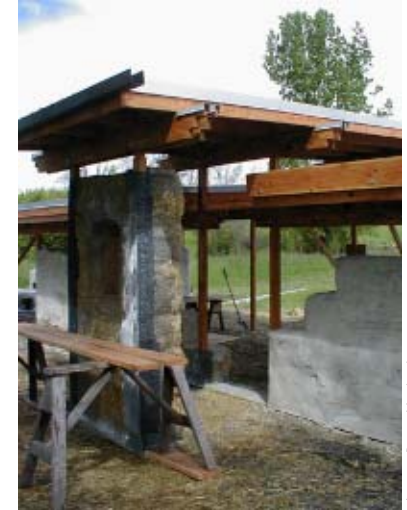
The PCEI bike shelter nearing the end of construction during finals week.
